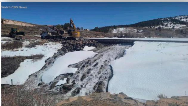
In this photo provided by the Utah Division of Water Rights, crews use heavy machinery to place boulders downstream of the cracked Panguitch Lake Dam to reinforce the wall on April 10, 2024.
